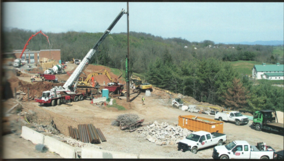
Work on the new academic building has begun on the site of the old maintenance building.
