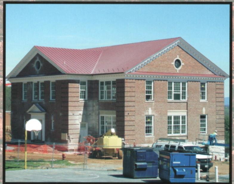
The renovations are nearly complete on the Stuart Building which will hold the a library media center on the top floor and the Student Center on the ground floor.
