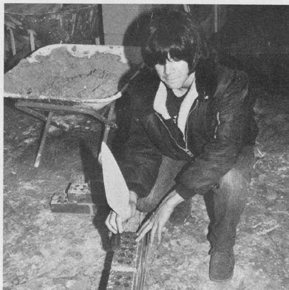
John Clark got the idea what it is like to be a bricklayer.
