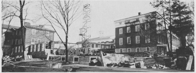
This picture was taken on January 10, 1935 during the construction of Perry Hall.
